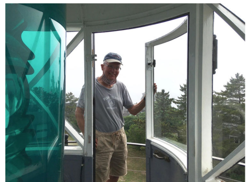
Board member Bill Cooper surveys repairs and supervises contractors from New England Glass and Finishing to repair cracked glass in the lantern room.
