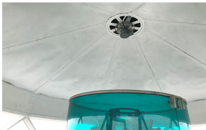
Ceiling of the repainted lantern room, painted by 2Penn Painting and Roofing in August 2020
