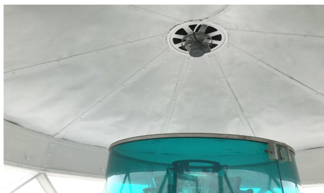
Ceiling of the repainted lantern room, painted by 2Penn Painting and Roofing in August 2020
